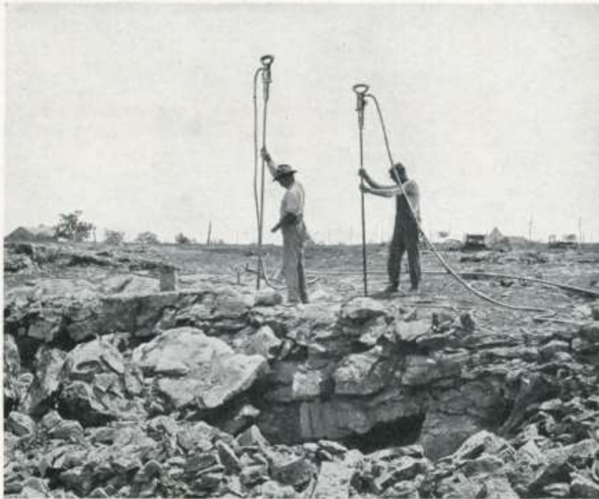
Sullivan "DB-19" hand feed hammer drills drilling holes eight feet deep, with hollow steel in quarry of Risley Bros. & Co., Jacksboro, Texas
