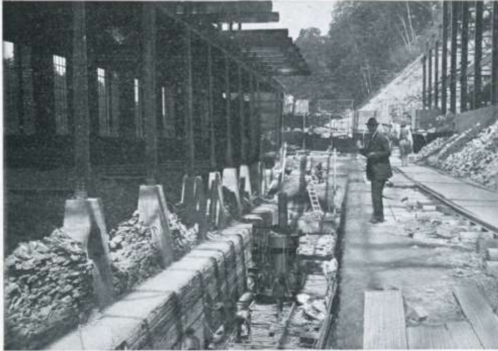
Condenser Wells, with Channeler at work
