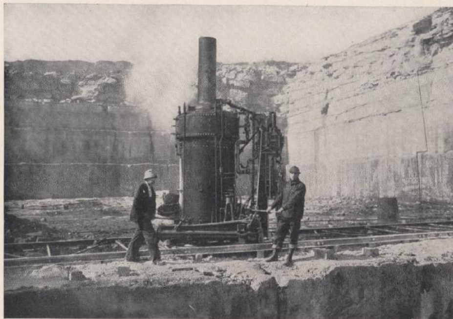
The Sullivan Duplex Channeler being swung on the turntable
