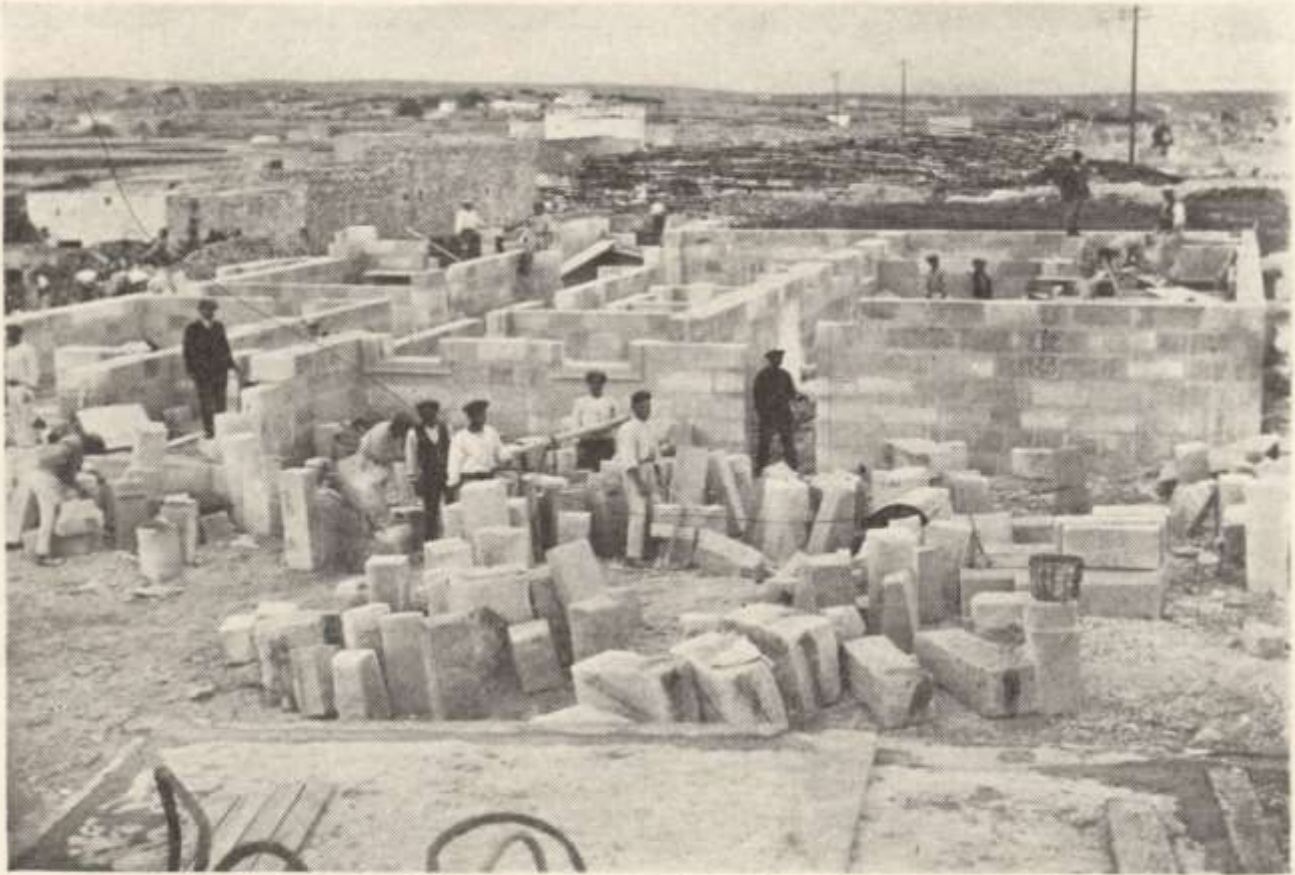
Erecting a Small House on Island of Malta, showing construction methods with walls rising from the ground level.
