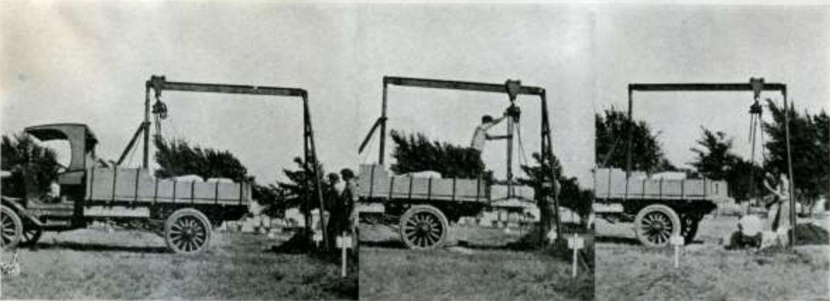
CUT NO. 4 SHOWS DEVICE RAISED AND ALL READY TO SET MONUMENT—SUPPORT REMOVED. NO. 5 SHOWS BASE IN AIR READY TO PLACE. NO. 6 SHOWS SETTING BASE IN PLACE. THIS DEVICE MAY BE USED OVER THE SIDE OF TRUCK OR AT ANY OTHER ANGLE.
